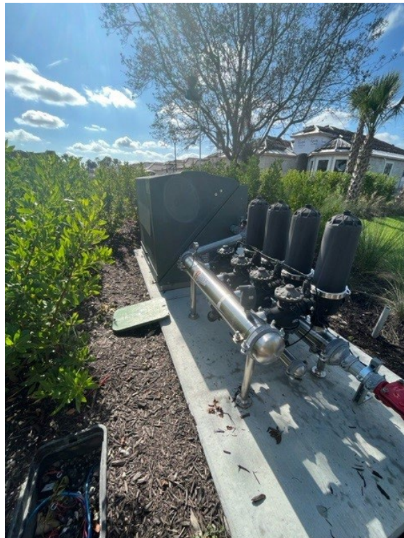
Irrigation - Pumps - Hatcher Parcel
