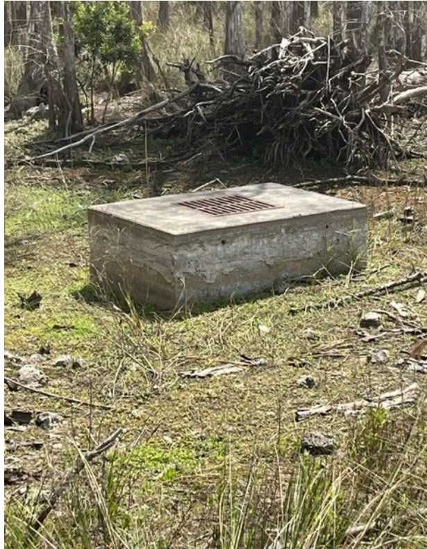
SWM – Bubble-Up Structure
