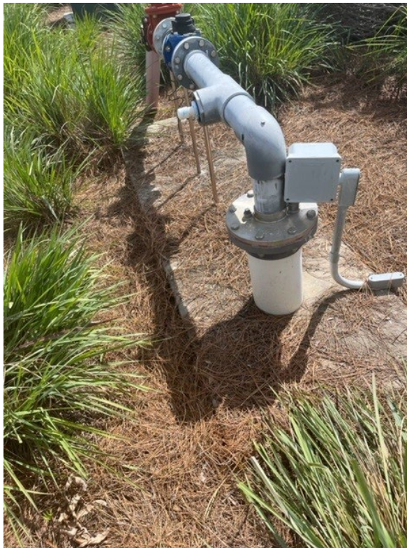
Irrigation - Recharge Well - Hole 12
